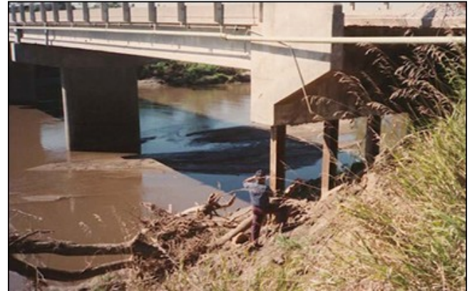
Fig. 1. A common case of abutment failure, where corrosion causes partial failure and soil seepage slope erosion [1].
